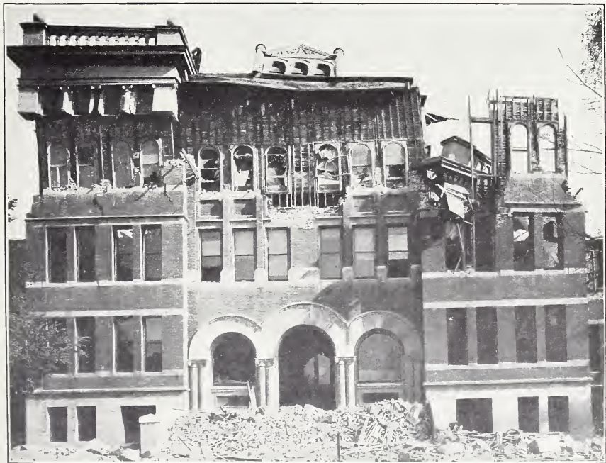
B. EARTHQUAKE EFFECT, HIGH SCHOOL BUILDING, SAN JOSE.
